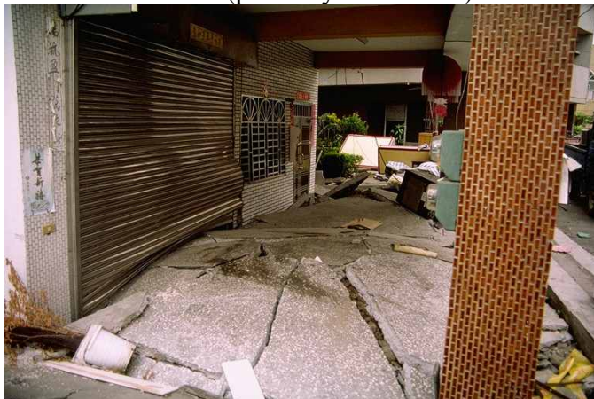
(c) Close-up view of foundation failures beneath a building [seen on left side of photo (a)] near the locations of borings WAS-3 and WAS-4 (photo by R. B. Seed)
