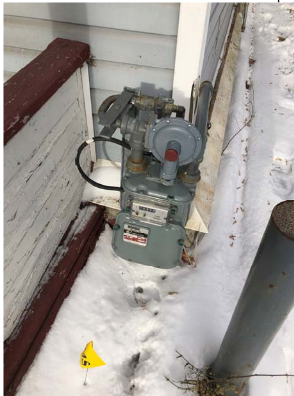
View of natural gas meter servicing site.
