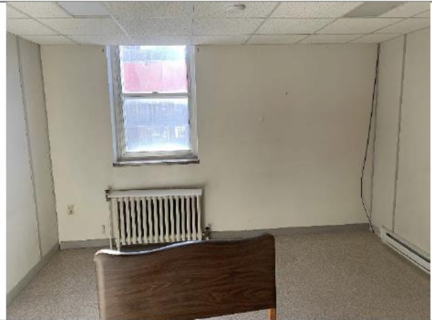
Figure 44: Empty office with sash window
