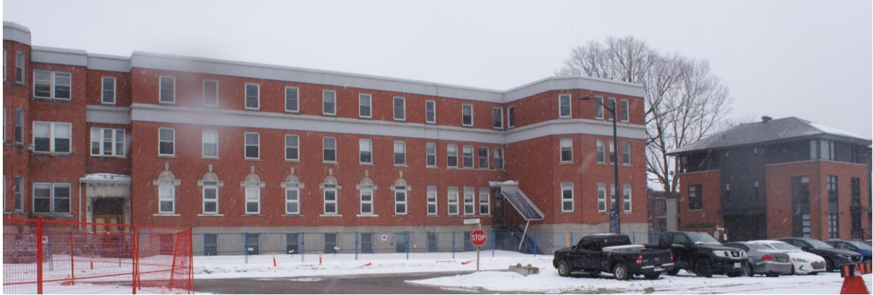
Figure 4: Partial view of the south façade to the east of the central bay. Source: Commonwealth
