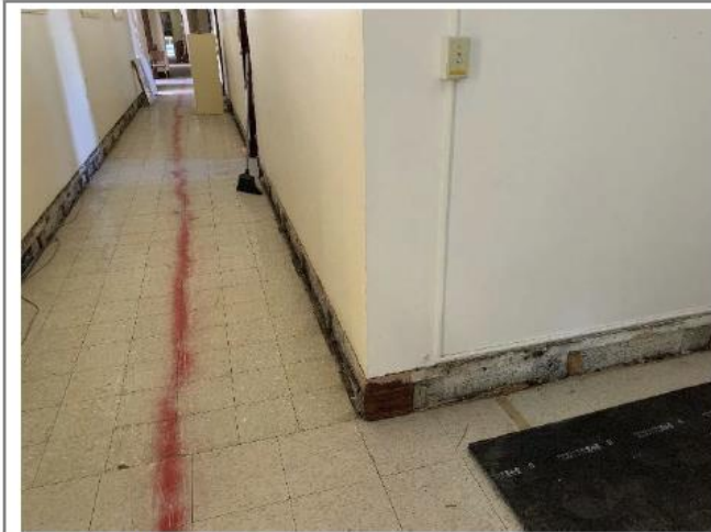
Figure 26: Extensive trim removals
