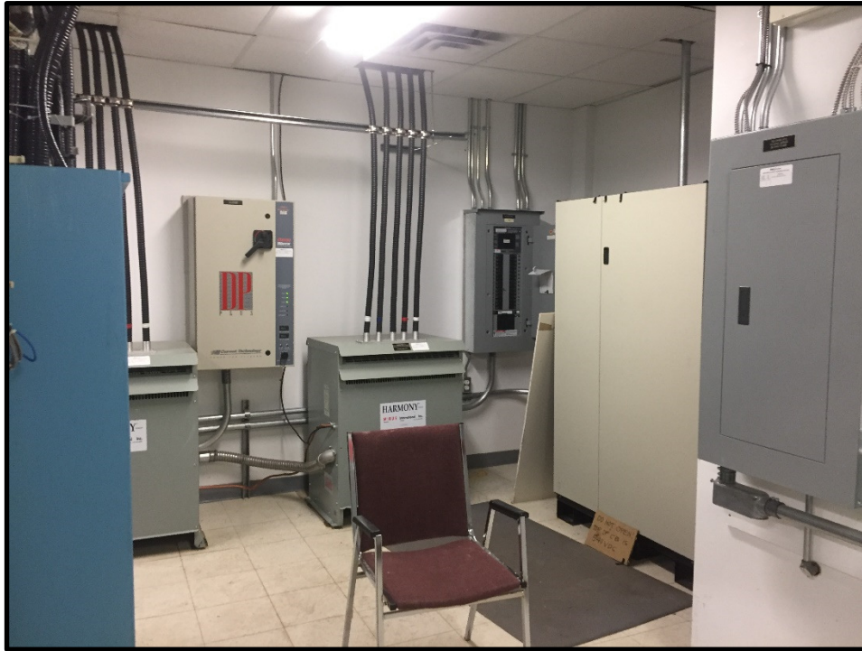
Photograph 3: Transformers within the building at 150 Laurier Avenue West.
