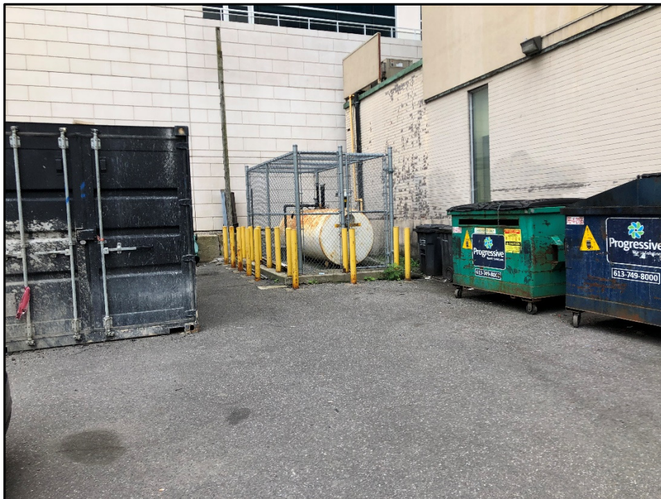
Photograph 2: AST observed at the exterior of 150 Laurier Avenue West.
