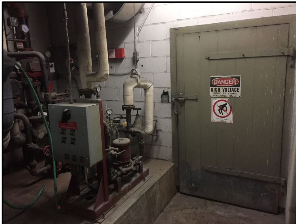
Photograph 4: Hydro vault within the basement of 150 Laurier Avenue West.
