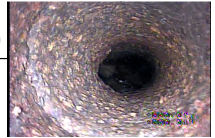
Figure#4: A view to the Surface Wear Large due to corrosion and grease at 1.6 meters from the top of the floor CO.
