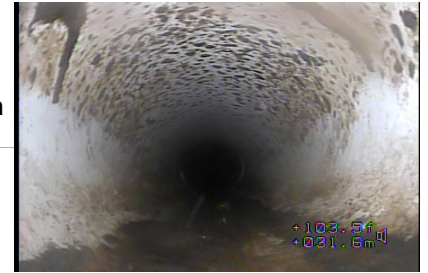
Figure#20: A view to the material change to PVC at 31.2 meters from the top of HALLWAY FLOOR CO.
