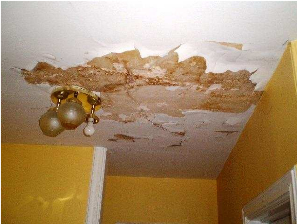
ceiling water damage - 2nd floor
