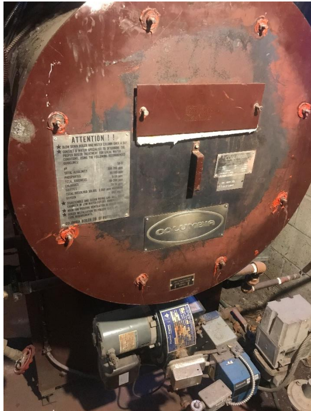
Photograph 28: Boiler in basement of Site building (April 6, 2021).
