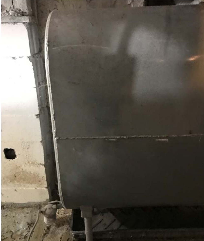
Furnace oil AST in basement
