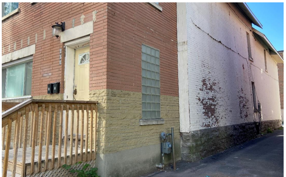
7 Close up of brick addition to the front of 230 Lisgar showing the connection between old and new. MTBA
