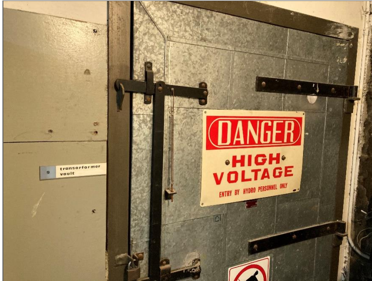
Photo 9 – Hydro vault located in the basement within the Site Building on the Phase One Property (PCA #1).
