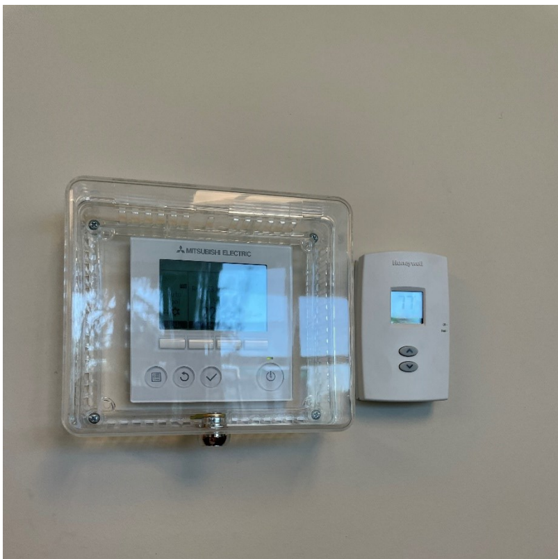
Photo 242: Typical thermostat in the building
