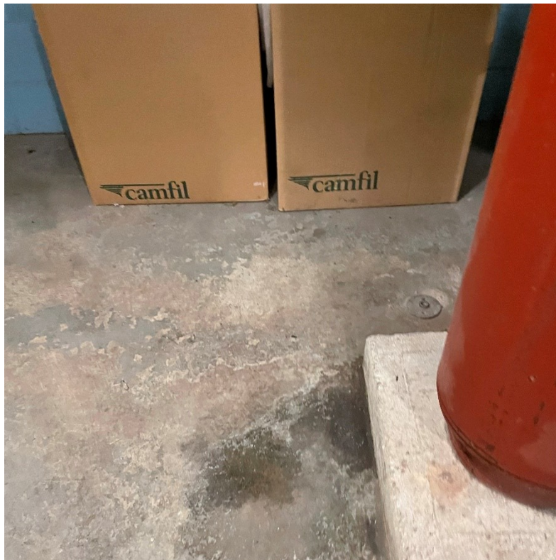
Photo 119: Evidence of historic leak in boiler room
