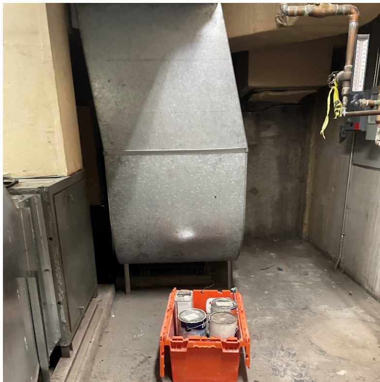
Photo 116: Paint storage in air handler room
