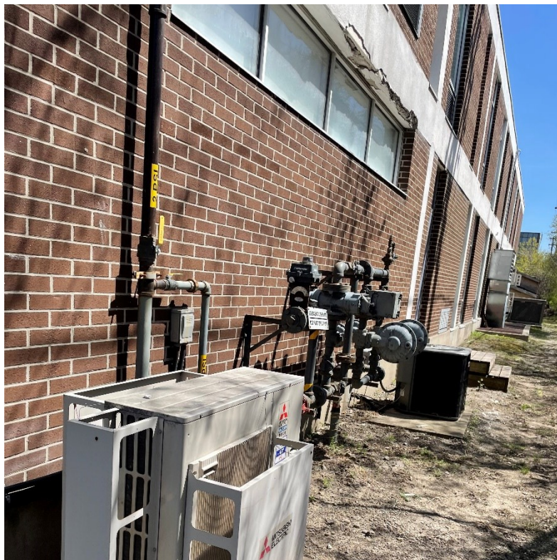
Photo 244: Outdoor mechanical equipment including air conditioning unit and the unsured hookup for backup generator
