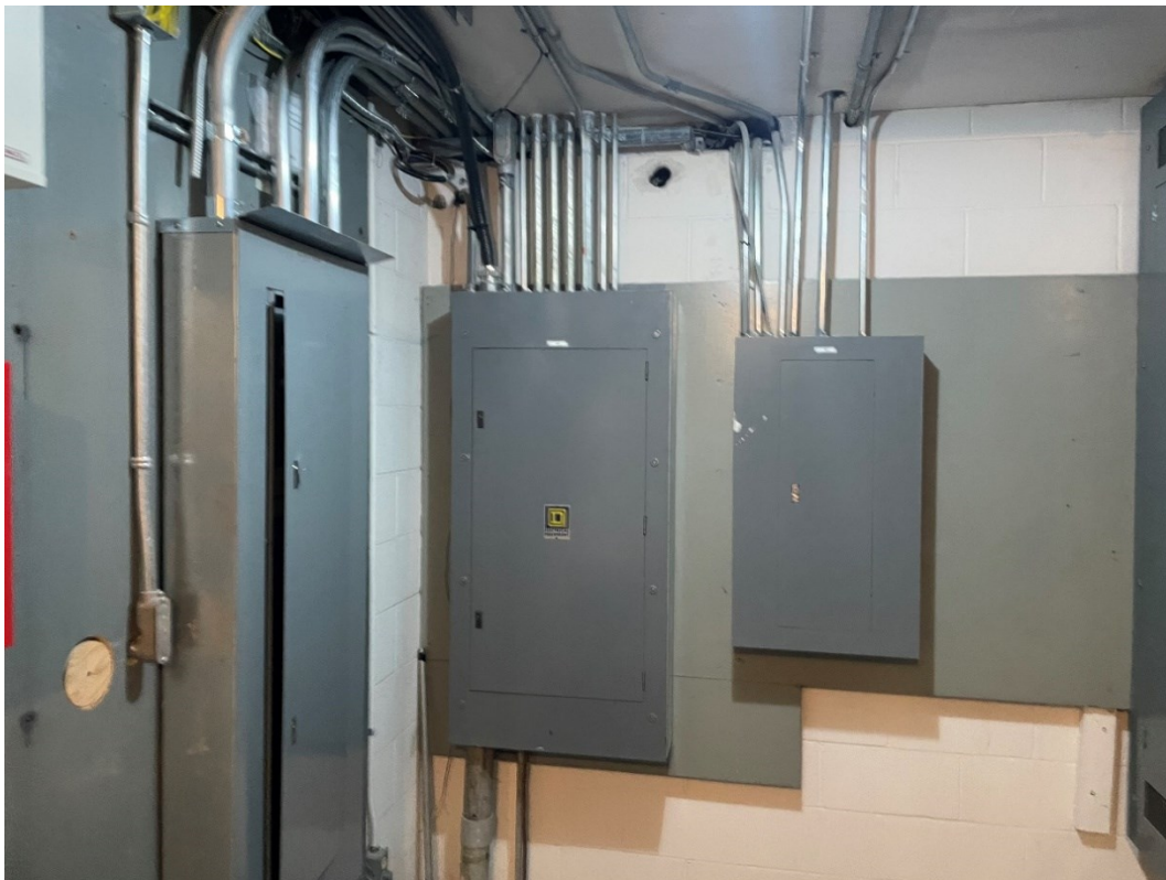
Photo 112: Electrical panels in air handler room
