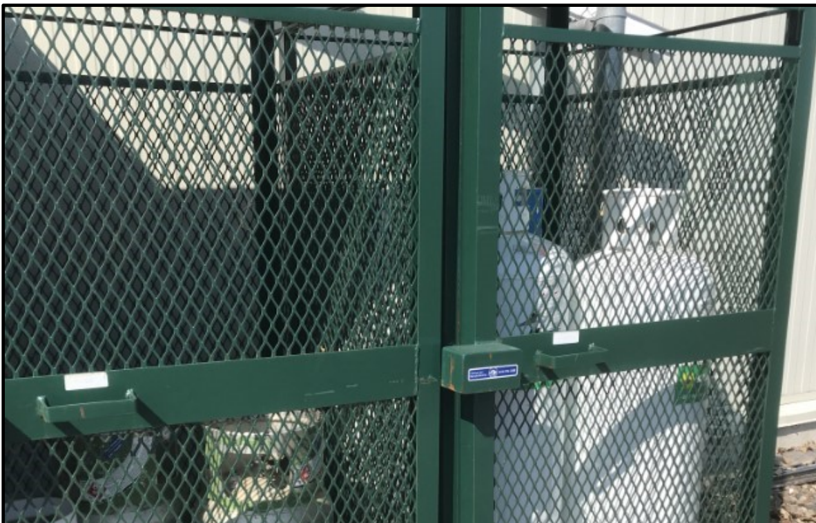
Photo 28: Photo of propane cylinders secured vertically in a storage cabinet to the east of the Site building.
