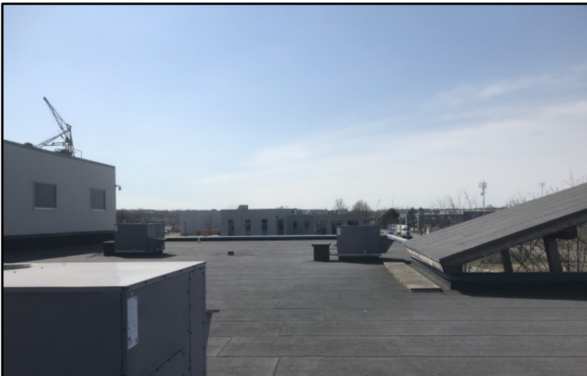
Photo 20: Rooftop view of four air handling units.
