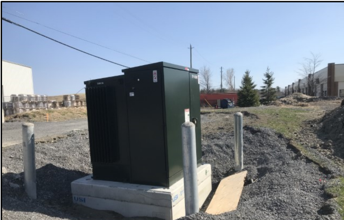
Photo 26: Pad-mounted transformer located on the north-boundary of the Site.
