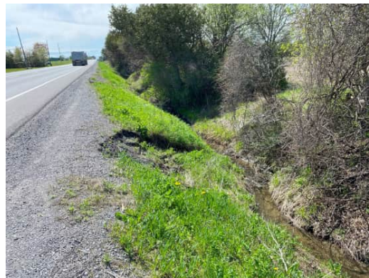
PICTURE 4: Shoulder Embankment Washout - Facing Southeast
