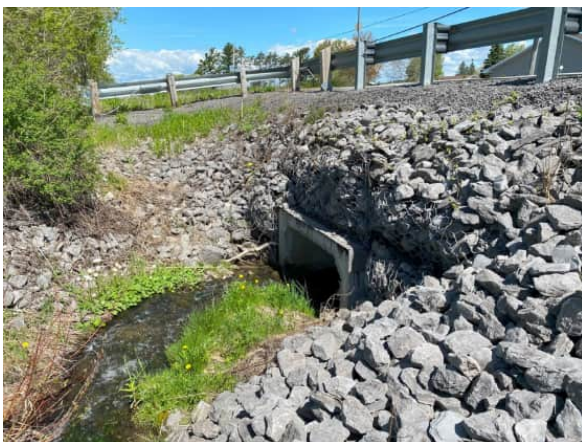
PICTURE 5: Large Box Culvert Crossing Carp Road 1.2km From Site - Facing North
