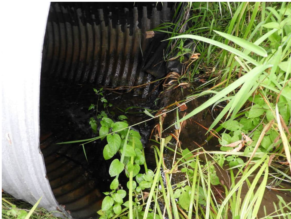
Photo 8: View of inlet of the culvert under Russ Bradley Road which conveys the tributary of Carp River from inside the study area to outside the study area. 11 August 2021.
