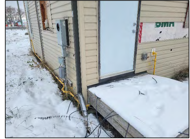
9. Photo is taken of the southwest corner of the trailer structure at 3497 Innes Road, showing the location of the utility connections, which were shut off at the time of the site visit.
