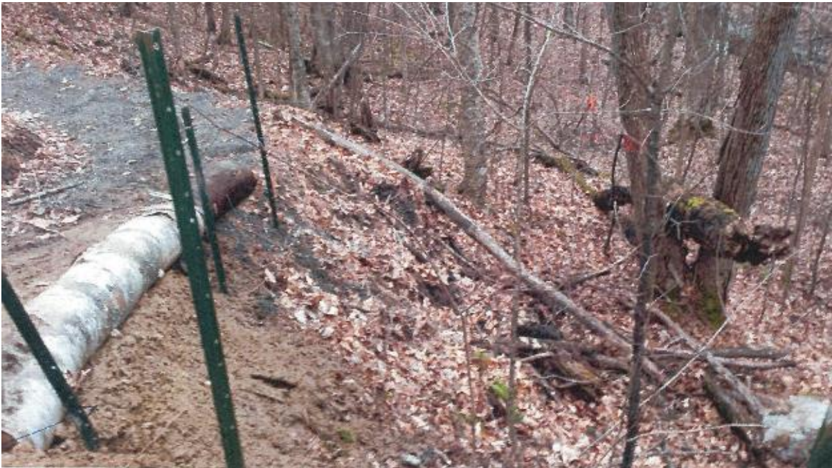
Photo No. 23 – Erosion of slope downhill of pathway. Area approximately 12 m long x 1.5 m to 2 m high.
