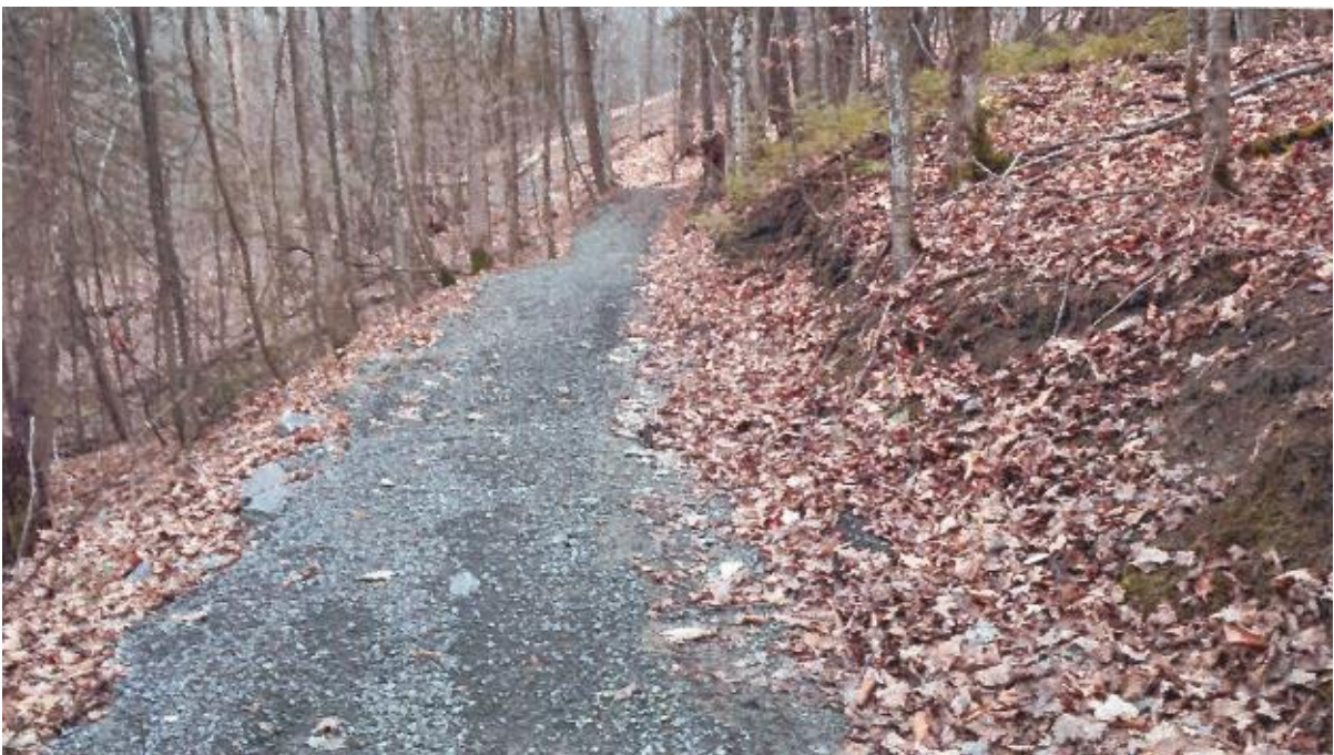
Photo No. 21 – Erosion of cut above pathway. Cut approximately 45 m long x 0.3 m to 0.8 m high.
