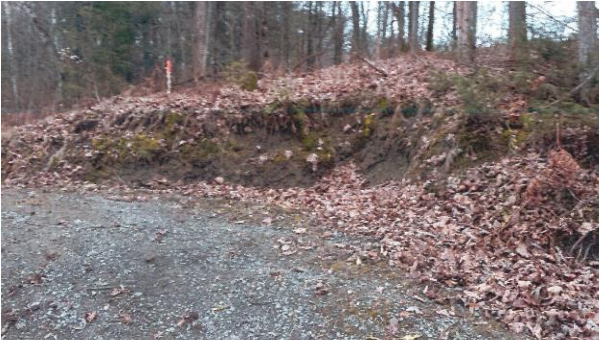
Photo No. 18 – Erosion of cut uphill of pathway. Cut approximately 3 m long x 1.2 m high.
