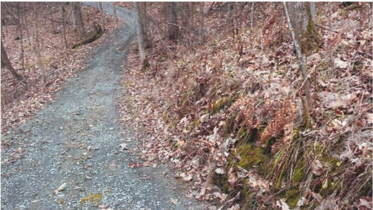
Photo No. 19 – Erosion of cut above pathway. Cut approximately 7 m long x 0.8 m high.
