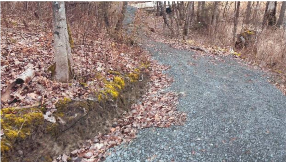
Photo No. 17 – Erosion of cut downhill of pathway. Cut approximately 30 m long x 0.3 m high.
