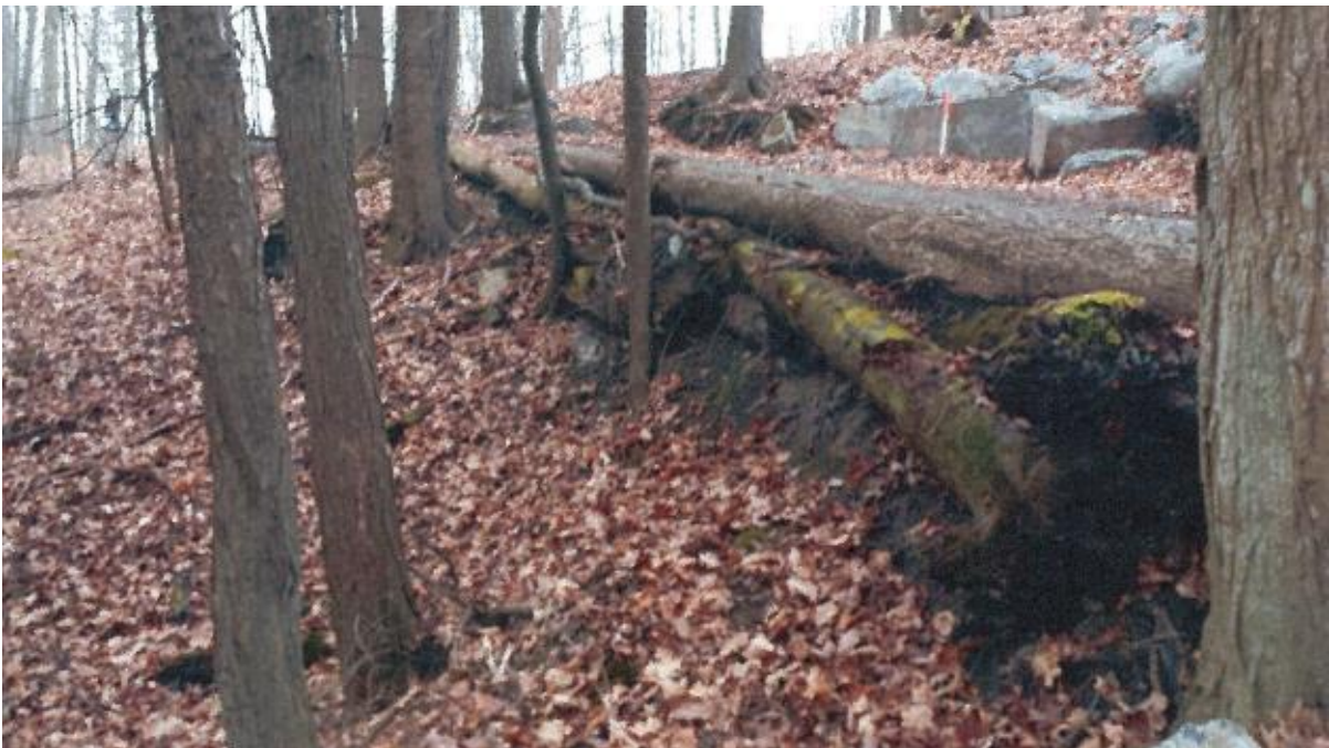
Photo No. 14 – Erosion of slope downhill of pathway. Note placement of logs to prevent erosion.
