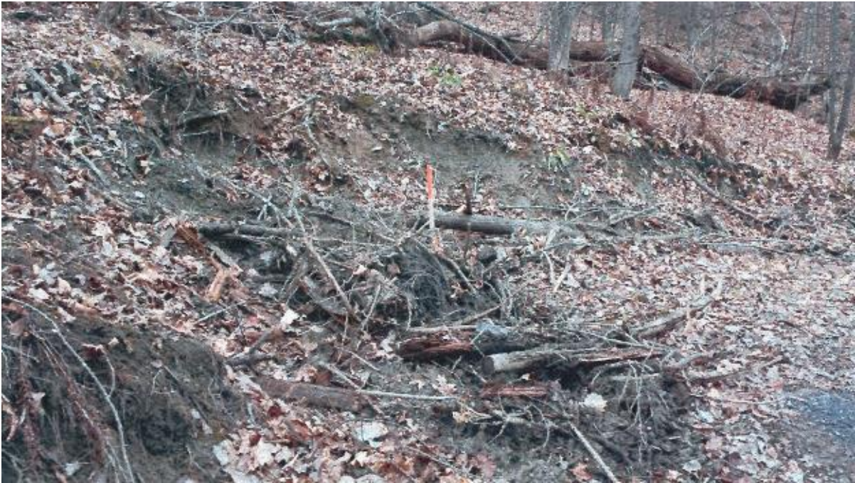
Photo No. 3 – Erosion above pathway approximately 5 m long x 0.4 to 1.0 m high
