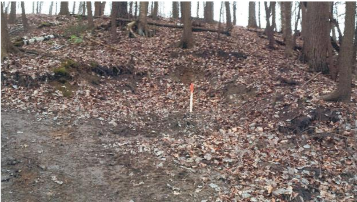
Photo No. 4 – Erosion above pathway. Approximately 3 m deep and 0.6 m to 1.3 m high.
