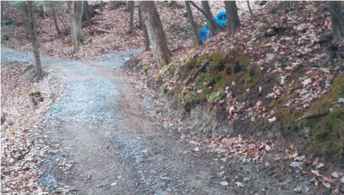
Photo No. 5 – Erosion of cut uphill of pathway. Cut approximately 12 m long x 0.9 m high.
