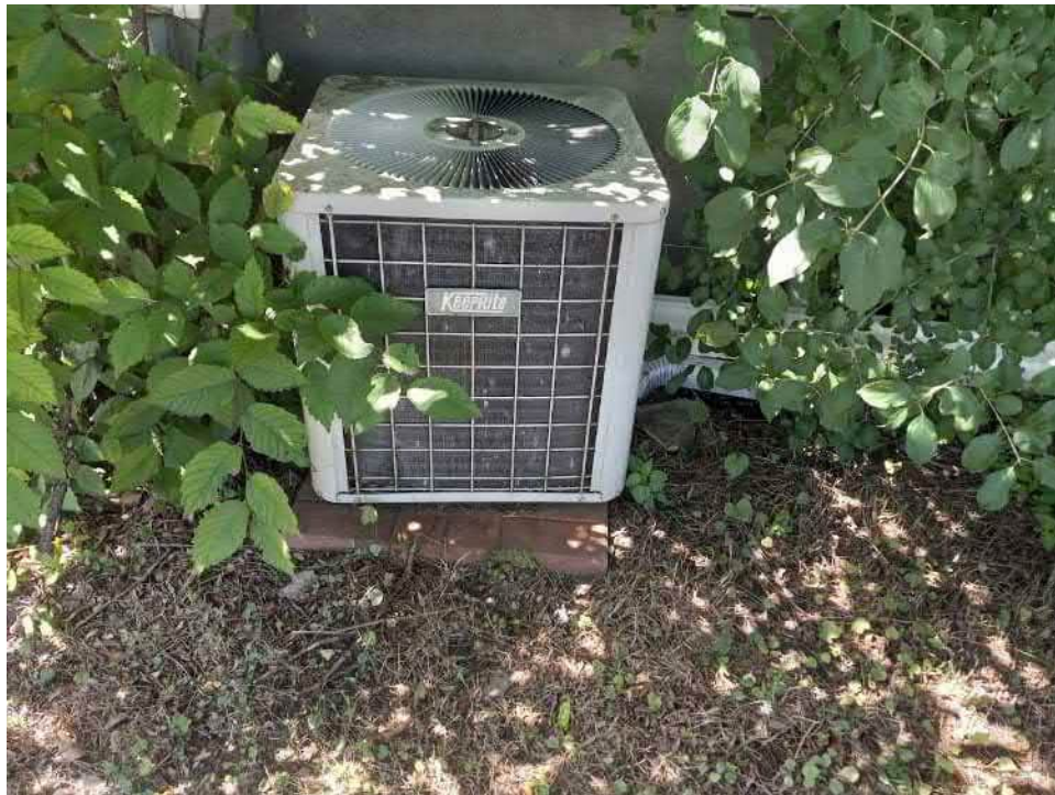
Photo 9: Air conditioning unit located alongside the eastern side of the building.
