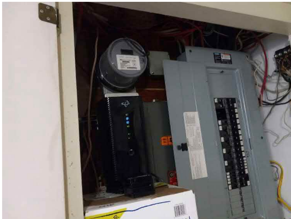
Photo 13: Electrical panel within one residential unit.
