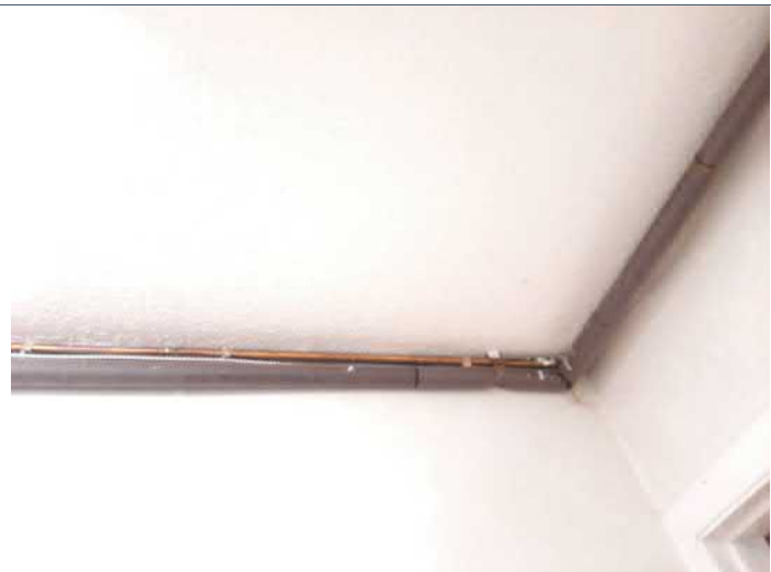
Picture 3 – Piping inside site building
