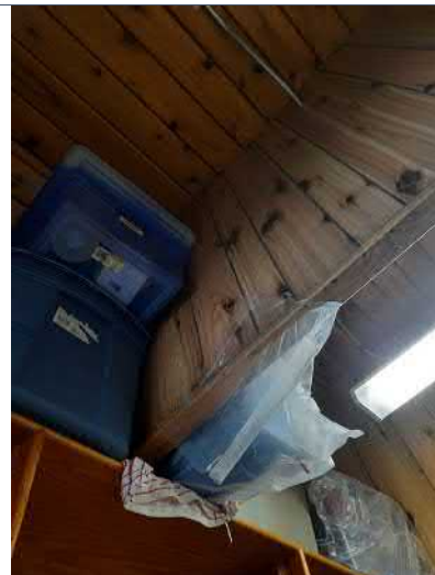
Picture 4 – Patched portion of ceiling in site building that has been reported by staff to have leaks in the past
