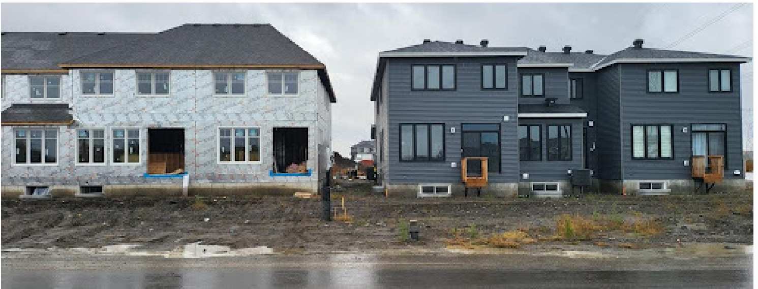
Photo #2 – Looking Southward from Cosanti Drive – rear yards of houses under construction.
