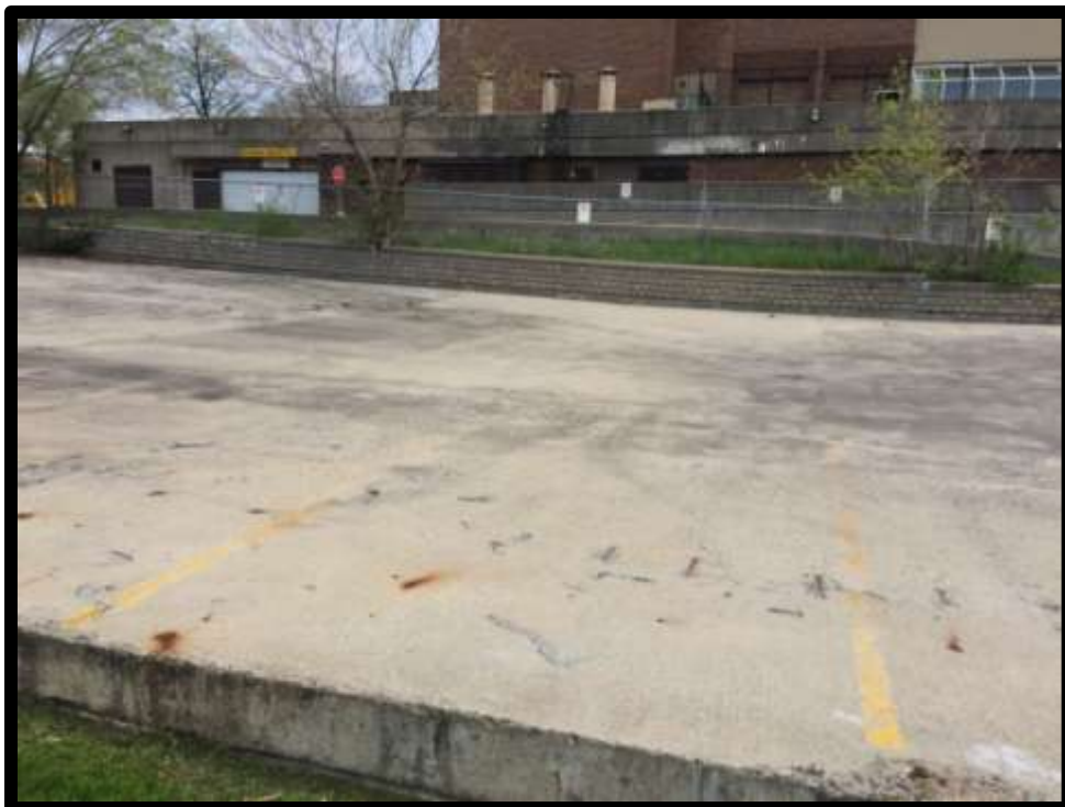
Photograph 4: View of upper level of the parking structure, facing south from the north side of the property.
