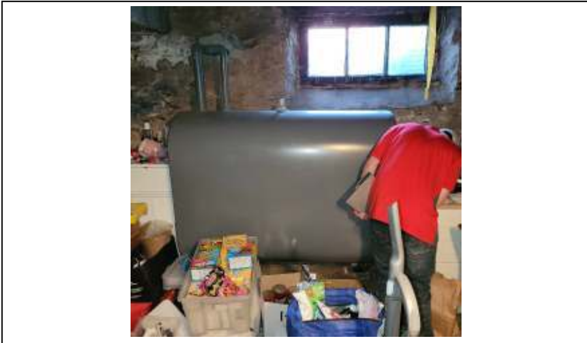
Photograph 23: 900 liter fuel oil aboveground storage tank in basement of 18 Hawthorne.
