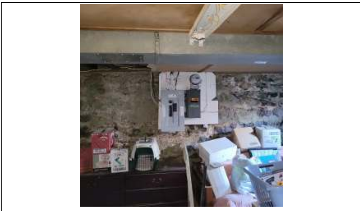
Photograph 10: Main electrical panel in basement of 12 Hawthorne.
