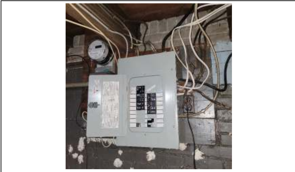
Photograph 7: Main electrical panel in basement of 14 Hawthorne.
