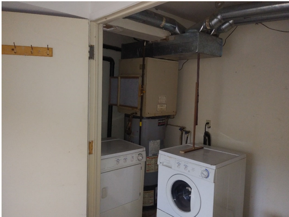
Photograph 8: View of one of the ground floor mechanical rooms in the residential building at the Phase One Property.
