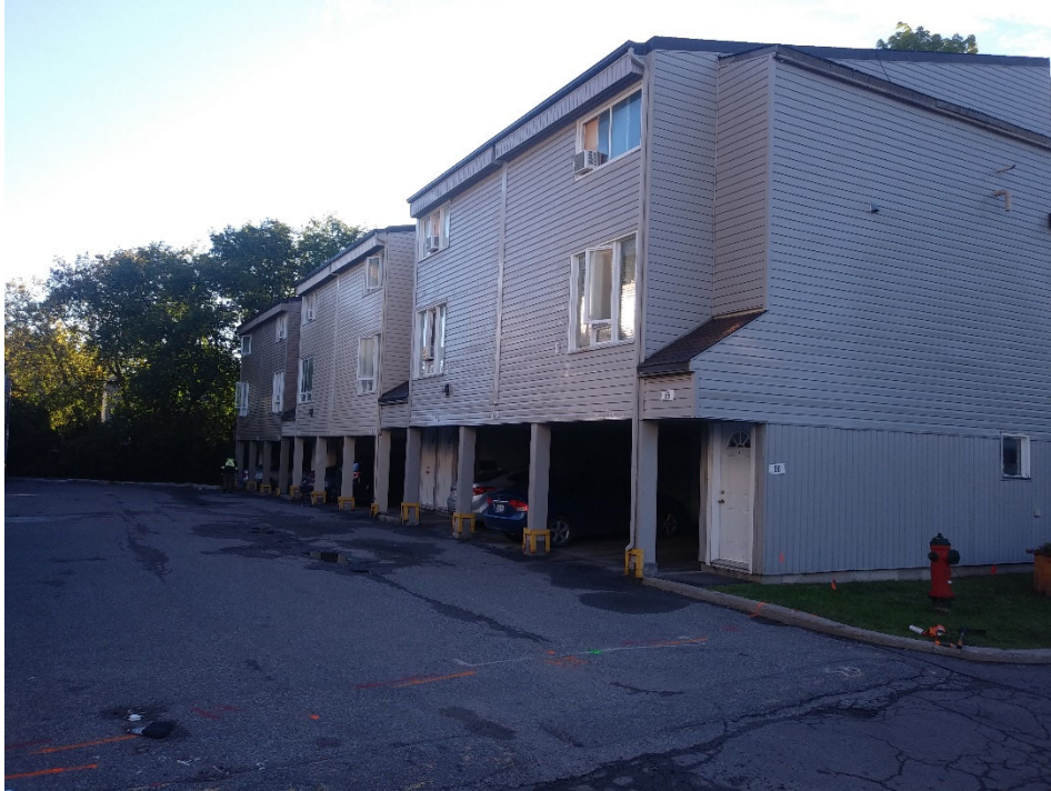
Photograph 1: View of residential building at the Phase One Property looking east-northeast from Finch Private (September 3, 2020).
