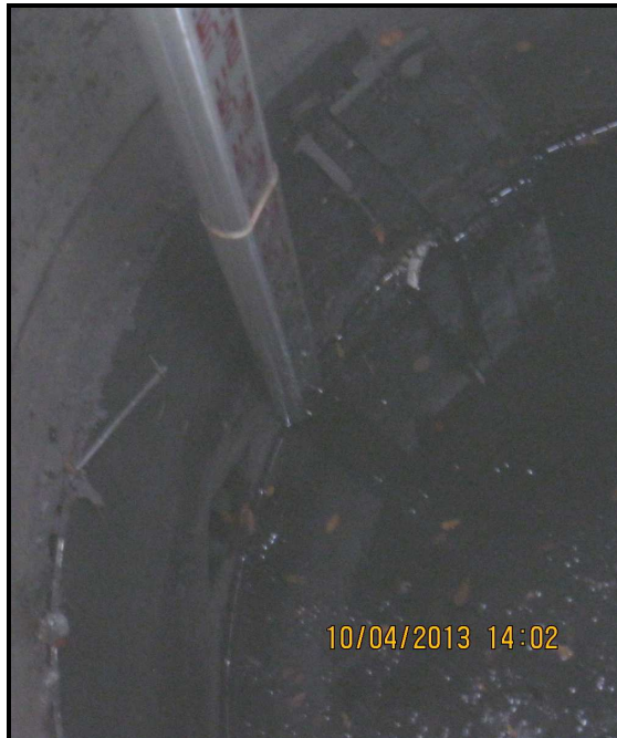
Figure 2a: Gate/Orifice in MH16
