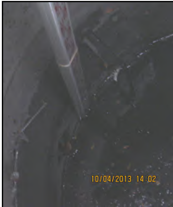
Figure 2a: Gate/Orifice in MH16
