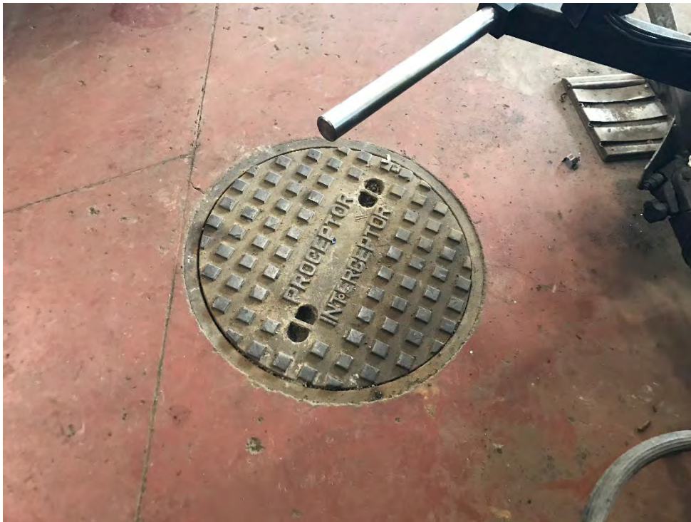
Photo 26 View of oil-water interceptor in the Automotive Service Centre. March 29, 2023.
