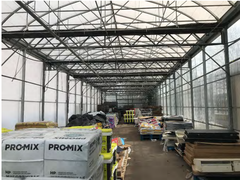
Photo 13 View of the fenced in Garden Centre at the southern portion of the Site. March 29, 2023.
