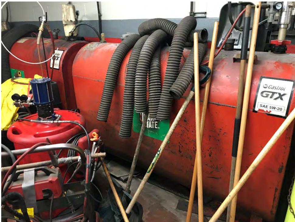
Photo 64 View of bulk oil tanks in the Automotive Service Centre. March 29, 2023.
