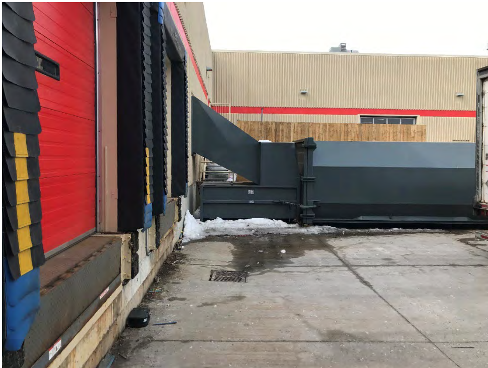
Photo 30 View of loading dock and catch basin located at the exterior of the Automotive Service Centre, facing west. March 29, 2023.
