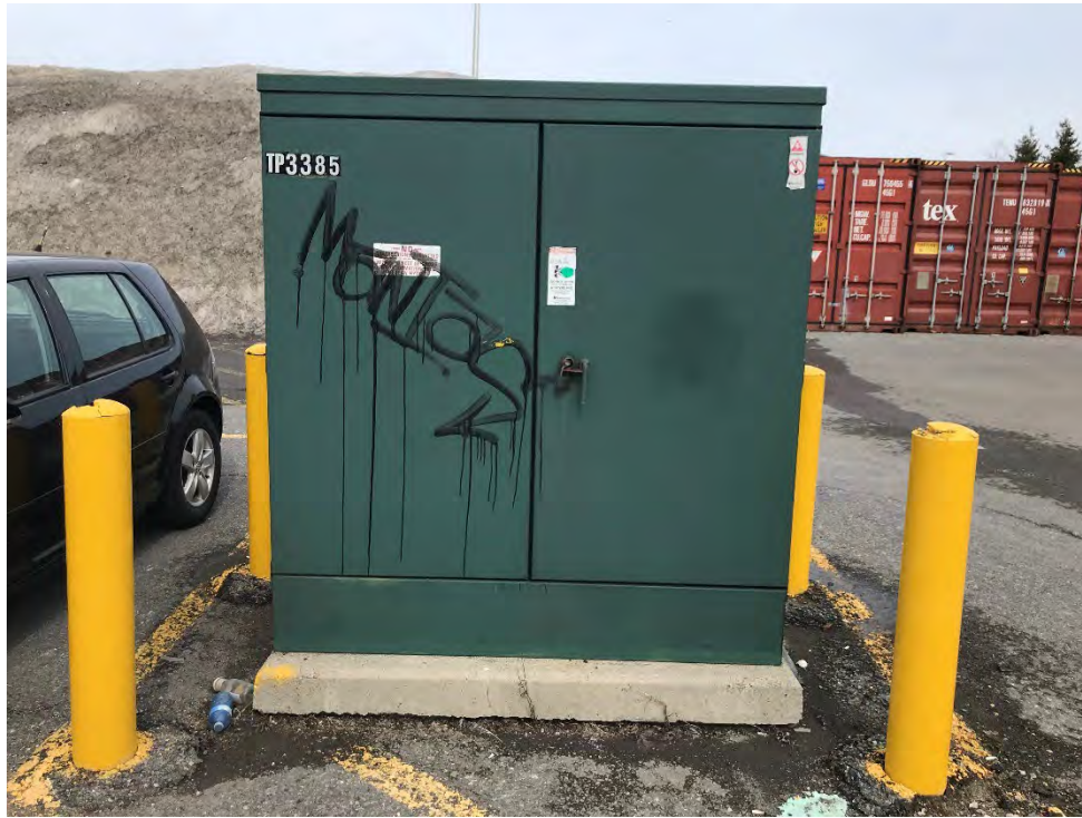
Photo 31 View of transformer located in the parking lot at the northern portion of the Site, facing north. March 29, 2023.
