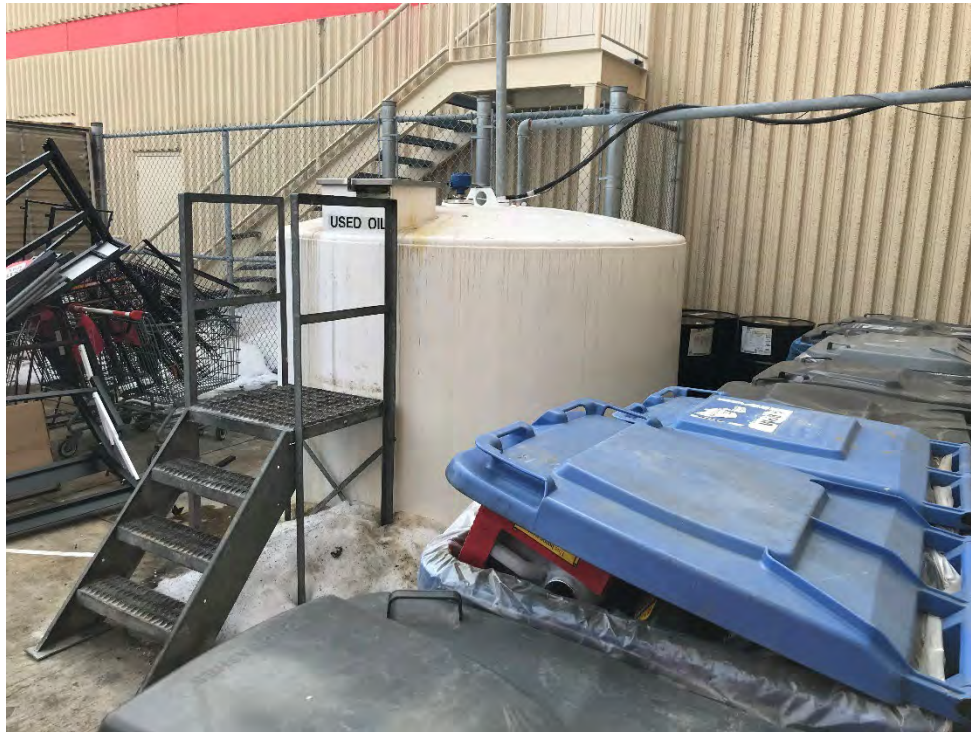
Photo 27 View of waste oil AST with a 3,000 L capacity located at the exterior of the Automotive Service Centre, facing southwest. March 29, 2023.
