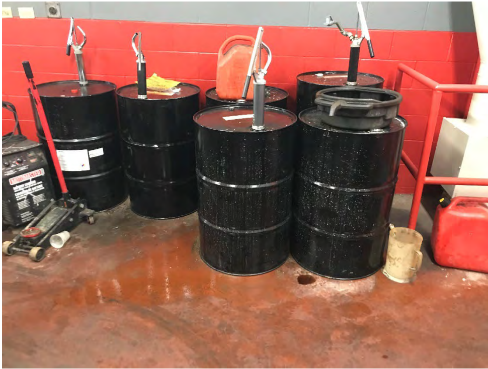
Photo 75 View of drums containing oil in the Automotive Service Centre. Staining/oily surface on the floor is visible. March 29, 2023.
