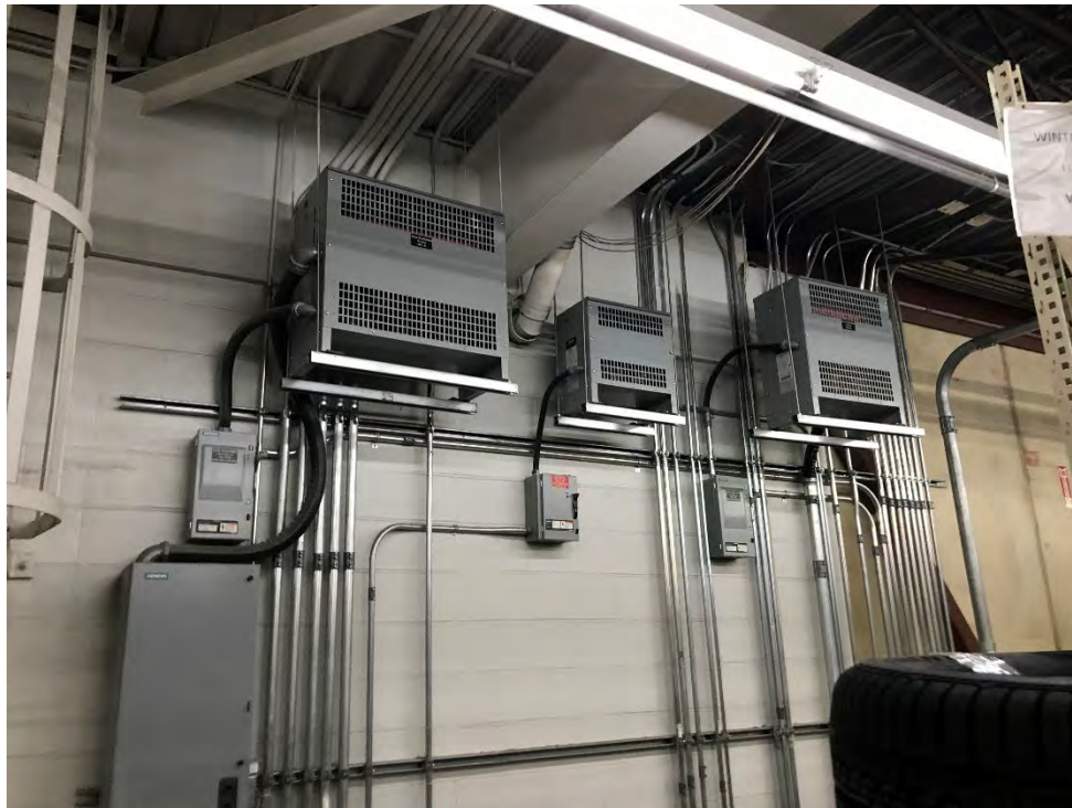
Photo 18 View of transformers located in the northeast corner of the Canadian Tire Warehouse. March 29, 2023.
