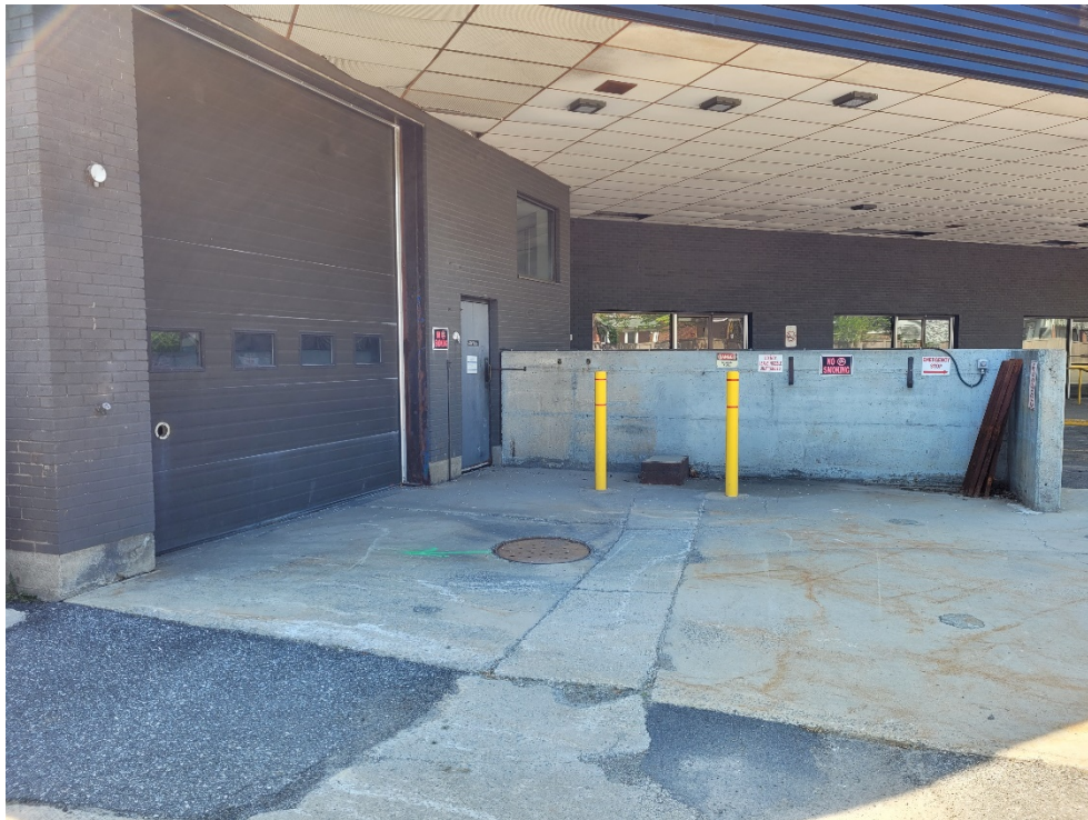
Photograph 4: View of the service garage entrance and former fueling area at the Property.
