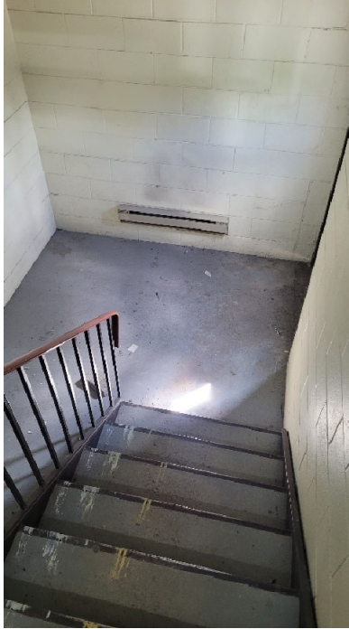
Photograph 7: View of the entry stairwell on the ground floor of the Site building. View also depicts auxiliary baseboard heating.
