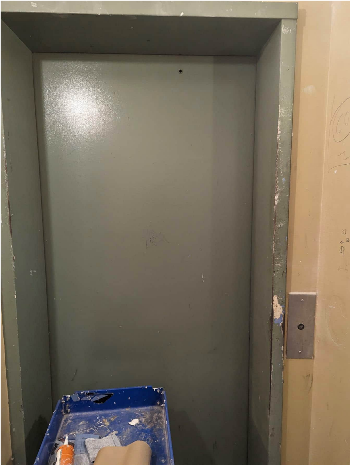
Photo 3: View of elevator within 1095 Merivale Road.
