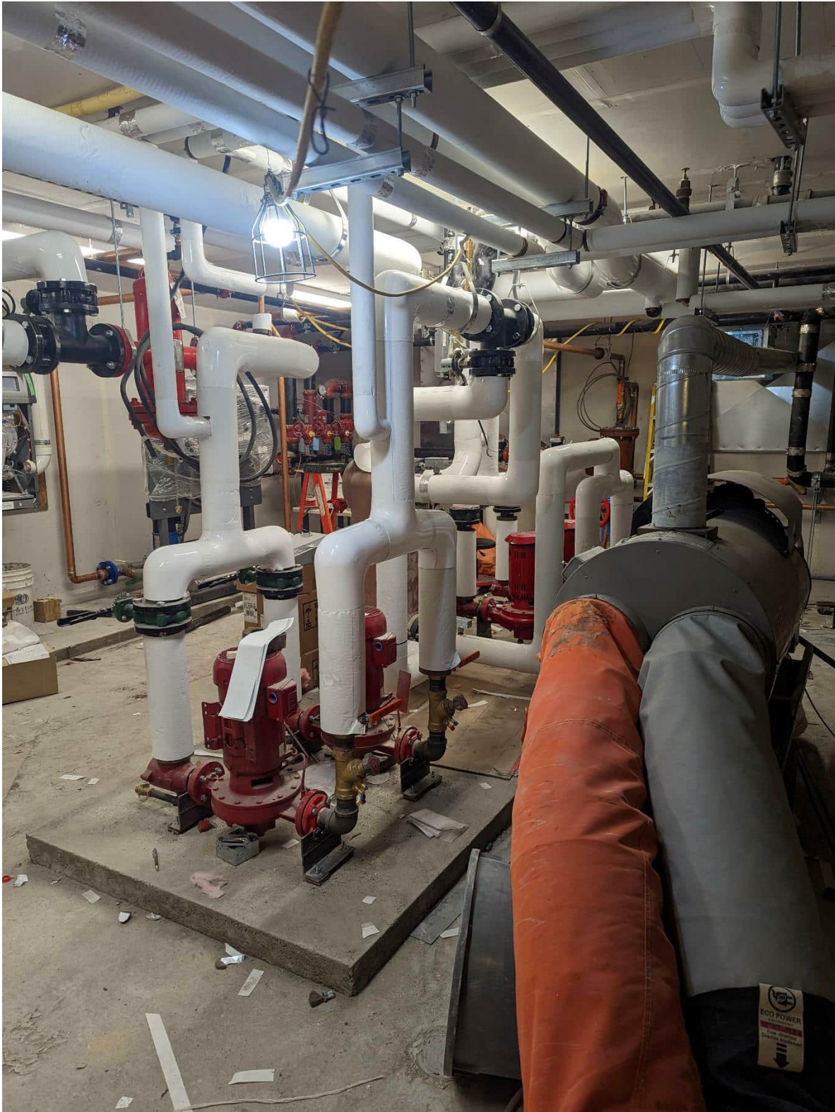
Photo 4: View of mechanical room within 1095 Merivale Road.
