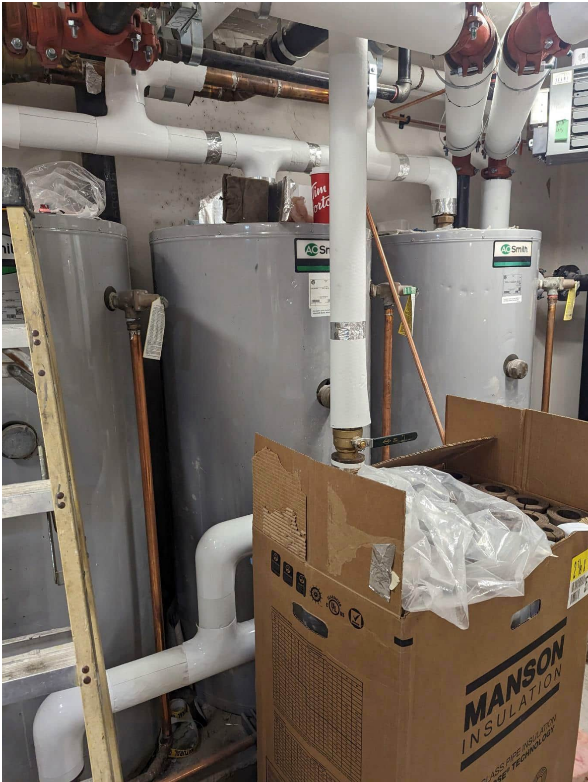
Photo 7: View of water heating system within 1095 Merivale Road.
