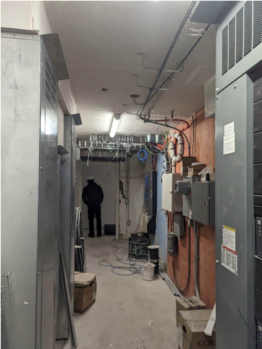
Photo 2: View of mechanical room within 1083 Merivale Road.
