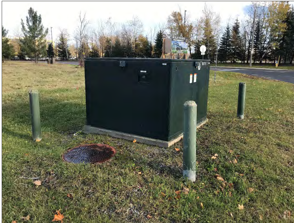
Photo 13: Transformer on southeast corner of Site. Date: 12/11/21 Direction: East
