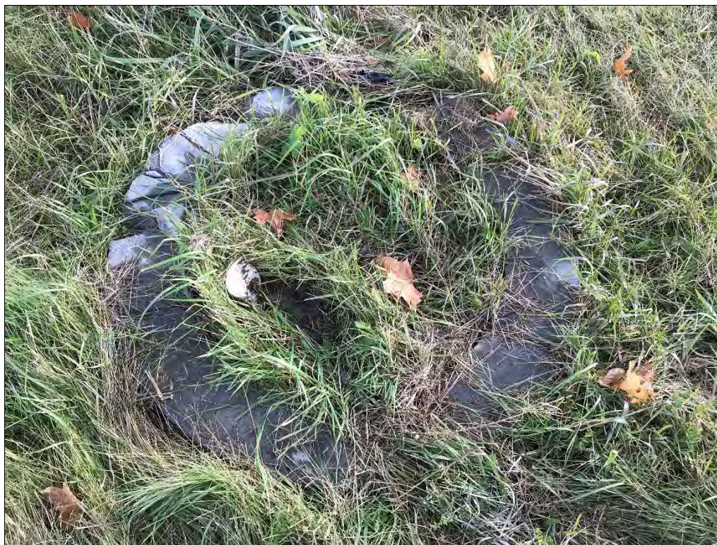
Photo 14: Unknown concrete "ring" on the southeast corner of Site. Date: 12/11/21 Direction: N/A
