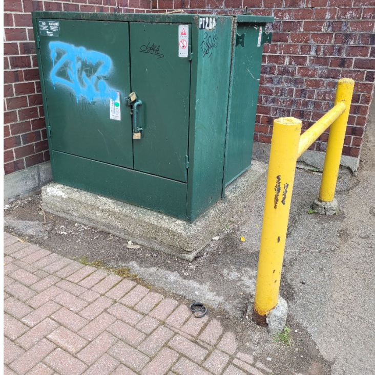
Photograph 9: View of the pad mounted transformer on the north portion of the Phase One Property.
