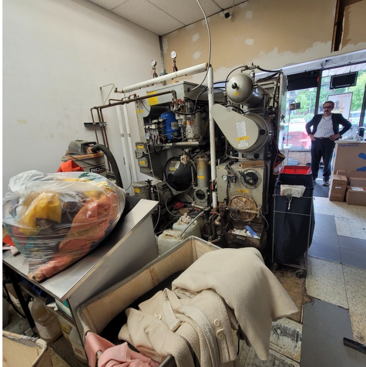
Photograph 5: View of the dry cleaning equipment on the interior of the dry cleaner unit. View is looking south.
