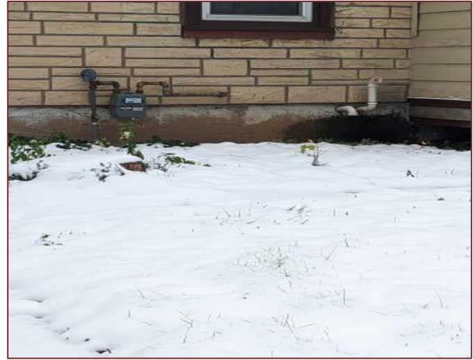
Photograph 10: Gas meter on front (north side) of home.
