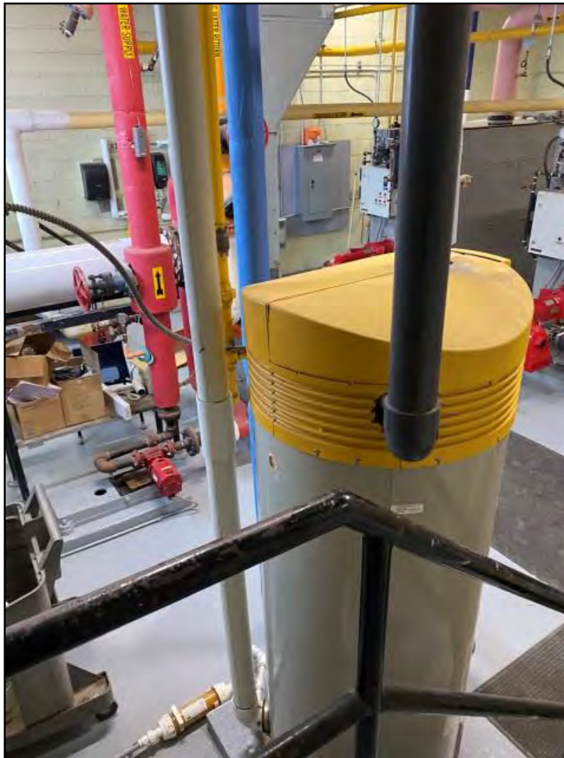
Photograph 8: View from the entrance of the boiler room. A hot water tank and various pipe systems are in view.
