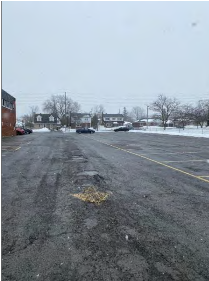
Photograph 25: Looking north at the parking lot on the west side of the school.
