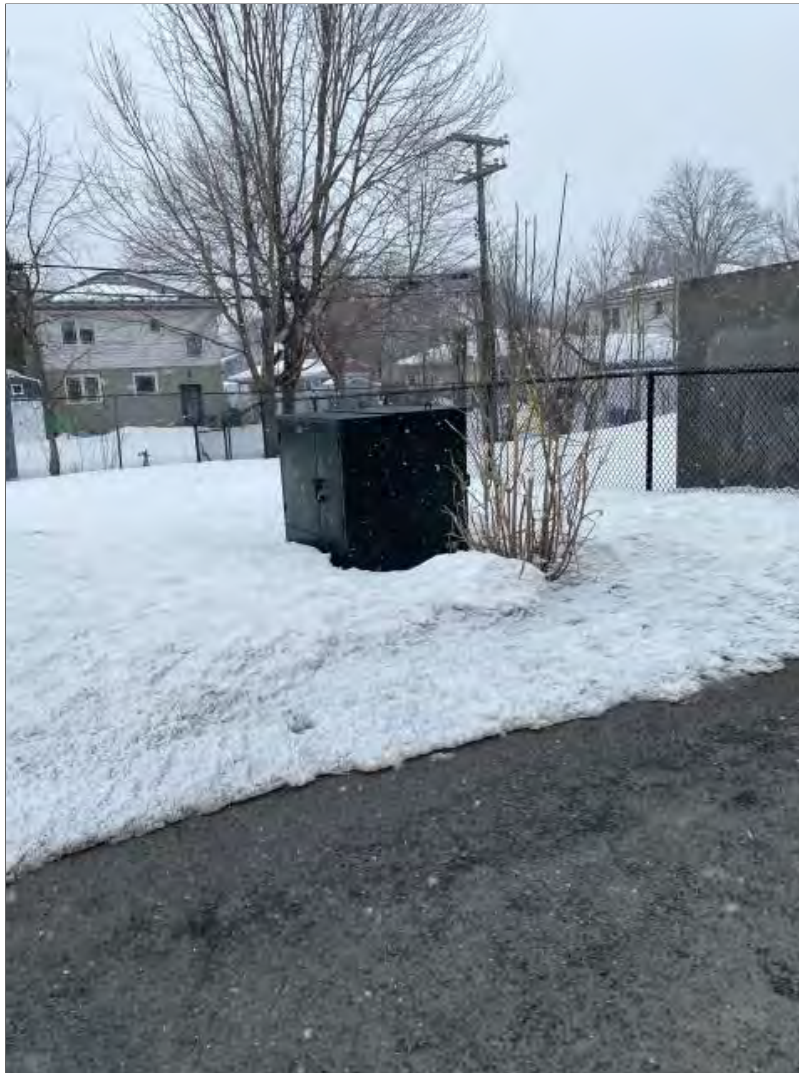
Photograph 26: Looking east at a transformer on the east side of the school. The second outbuilding is in view on the right side of the photo.
