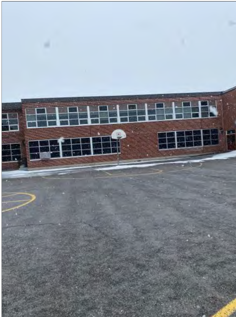
Photograph 21: View of the playground area. The exterior north wall is in view.
