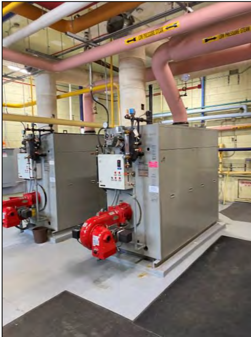
Photograph 15: General view of the boiler room.
