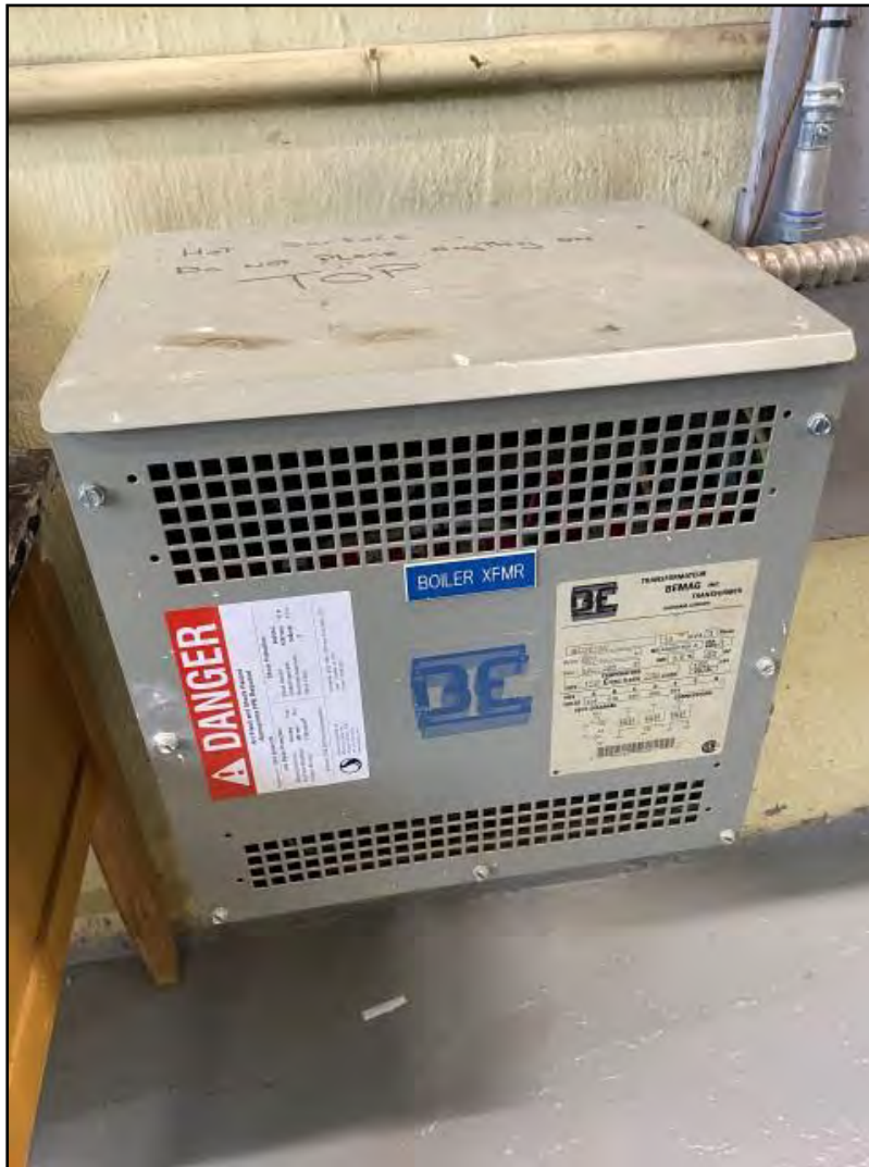
Photograph 13: View of the wall mounted transformer in the boiler room.
