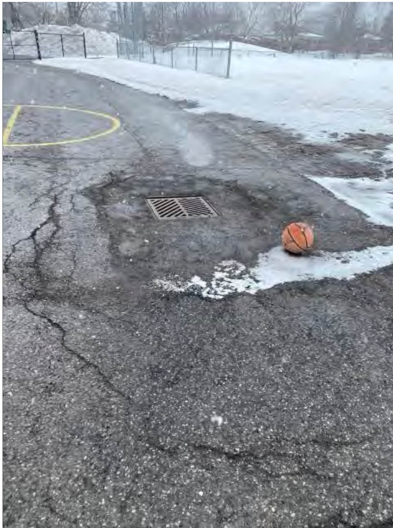
Photograph 22: View of the stormwater catch basin on the north side of the school.
