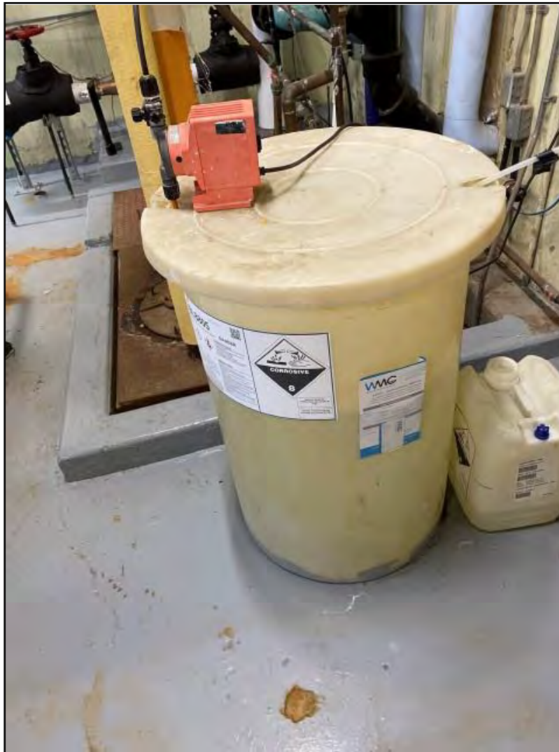
Photograph 11: View of a boiler water treatment tank.
