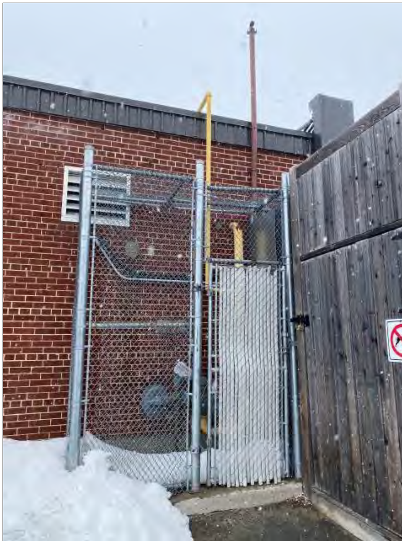
Photograph 27: Looking west at the natural gas meter on the exterior east wall of the school. What looks to be a vent pipe for a storage tank is in view.
