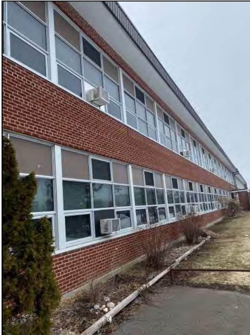
Photograph 3: Looking north-east at the exterior south wall of the building. Air conditioning units are in view.
