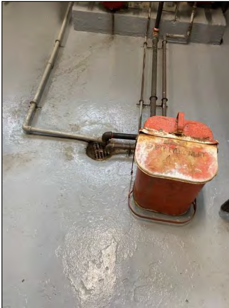
Photograph 14: View of another floor drain in the boiler room with condensation pipes.
