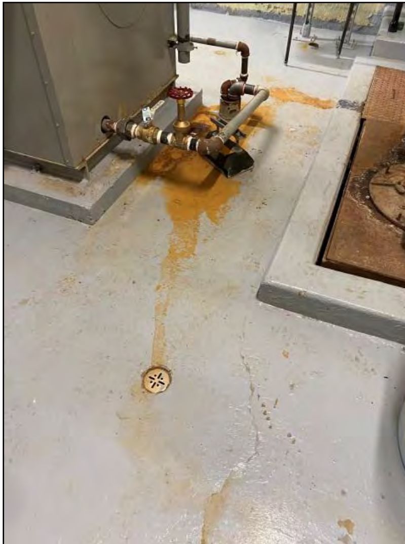
Photograph 9: View of a floor drain in the boiler room. Staining observed.
