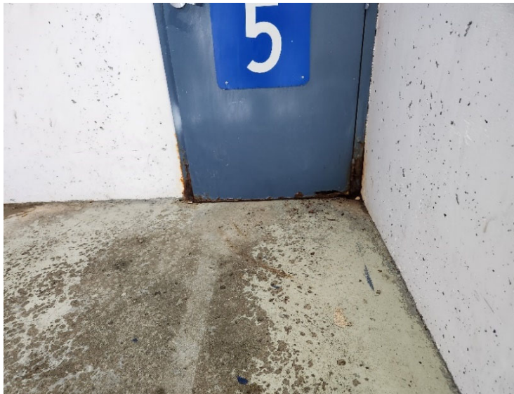
Photo 12 - Rusting/corroding door frame
