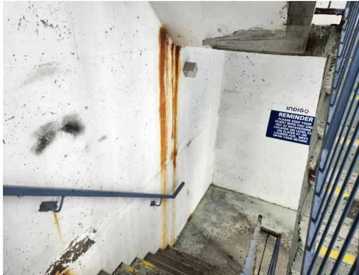
Photo 13 - Rust staining on stairwells
