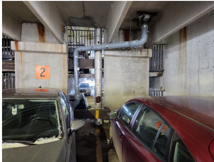
Photo 14 - Storm drainage piping
