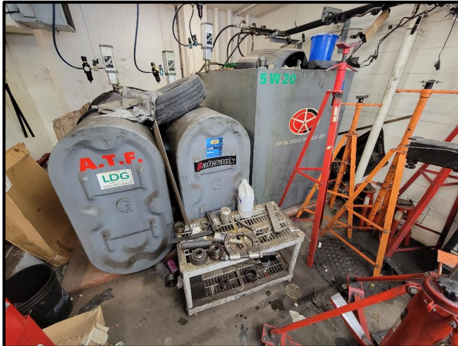
Photograph 8: View of three aboveground oil and transmission fluid storage tanks, and an oil/water separator (bottom right), located inside the vehicle maintenance garage in the northern portion of the Phase I Property.
