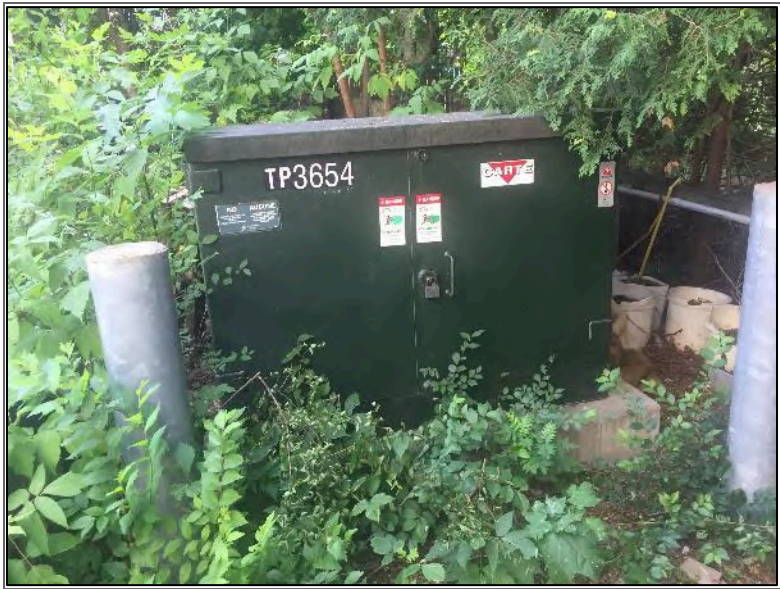
Photo 9 – Pad-mounted transformer located on the east portion of the Phase One Property.
