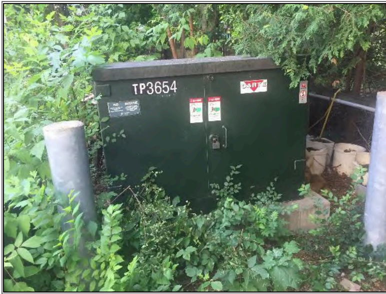
Photo 9 – Pad-mounted transformer located on the east portion of the Phase One Property.
