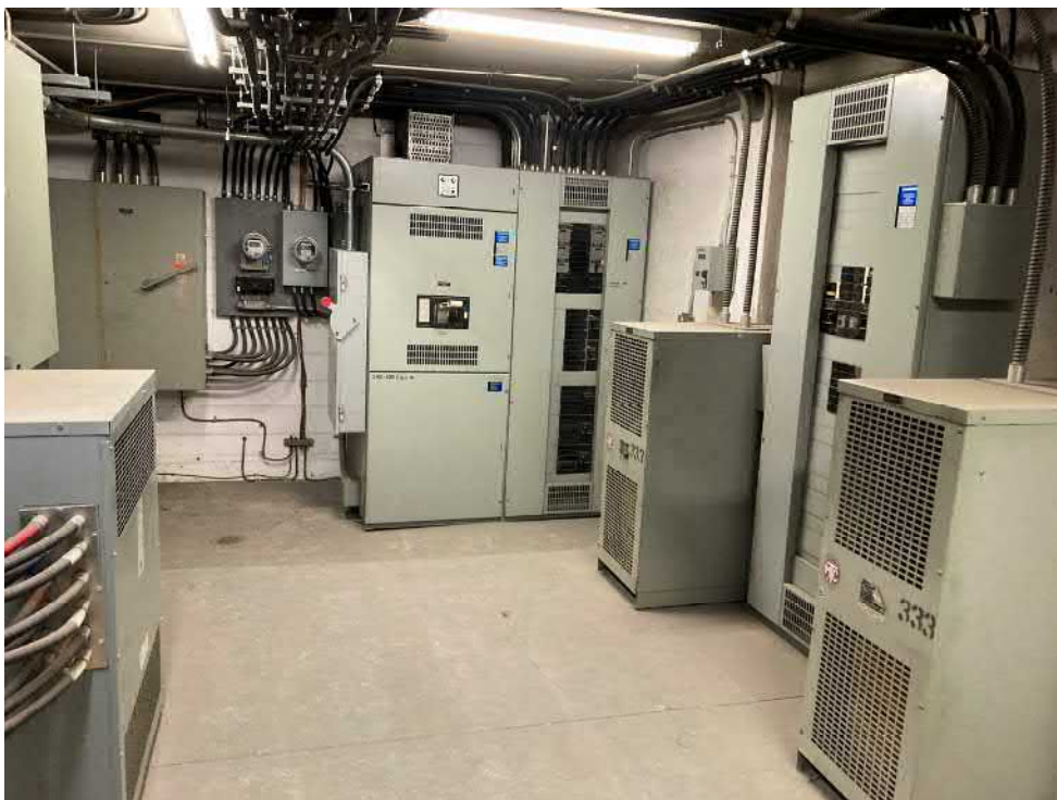
Photo 12: Basement electrical room
