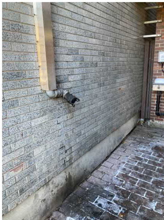
Photo 18: Foreground: grease trap cleanout pipe associated with Clocktower Brew Pub (food grease); vent and fill pipes for diesel generator at adjacent building to north in background
