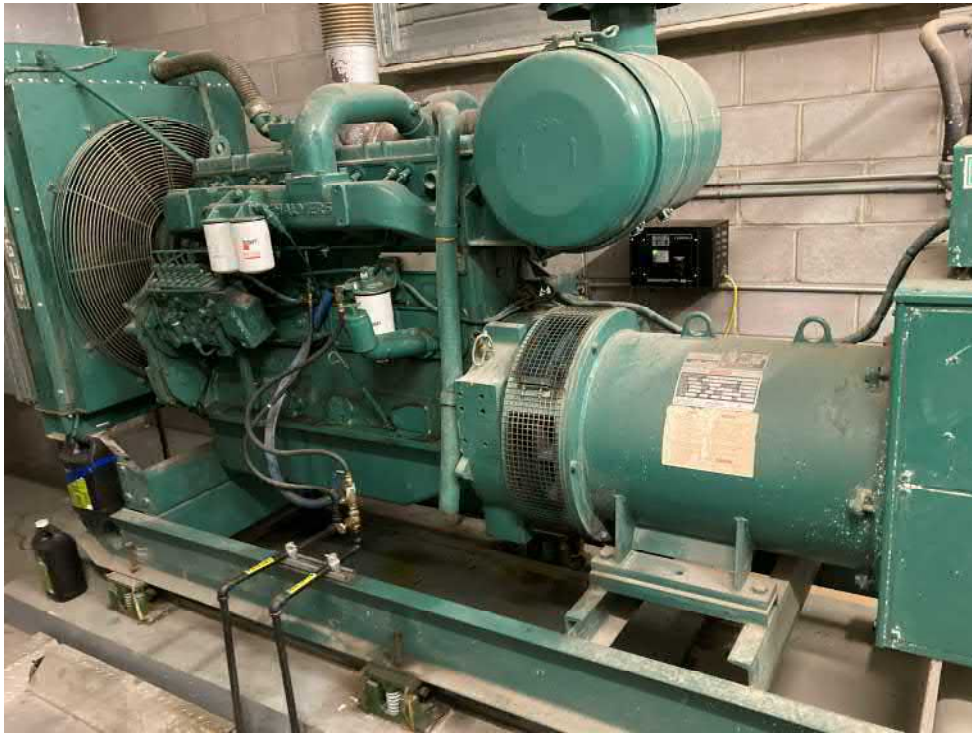
Photo 15: Diesel backup generator in mechanical penthouse (11 th floor)
