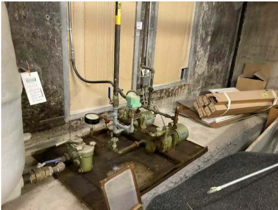
Photo 10: Pumps associated with diesel tank to bring diesel to generator on 11 th floor
