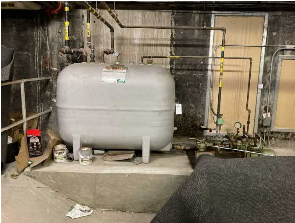
Photo 9: AST containing diesel fuel for backup generator. Tank is in basement mechanical room.
