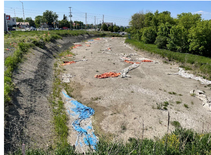
Looking north across the site from the southern boundary at the excavation area
