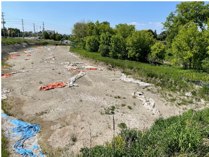
Looking northeast across the site from the southern boundary at the excavation and wooded area remaining
