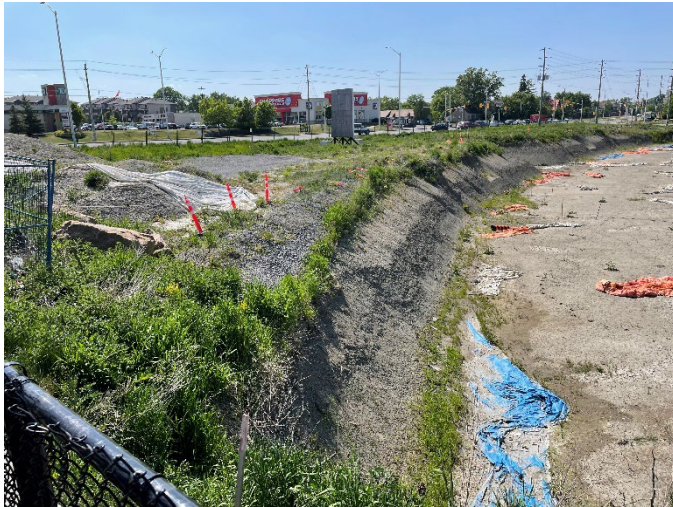
Looking northwest across the site from the southern boundary at the excavation and elevation change
