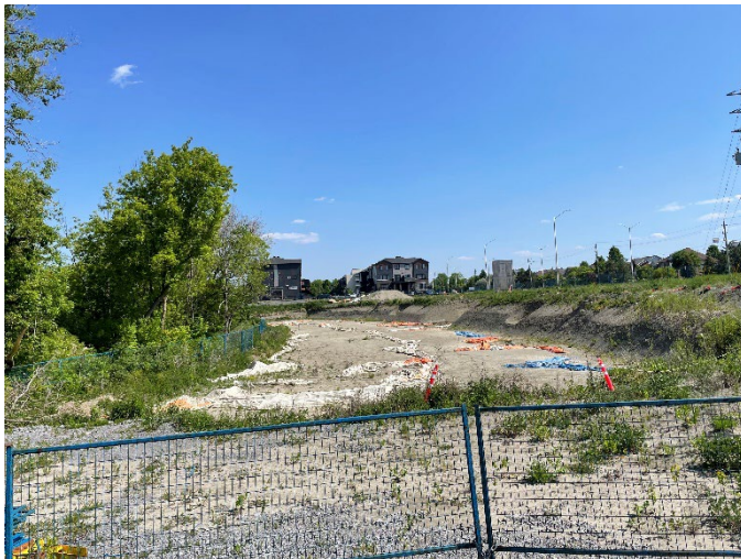
Looking south across the site from the access road along Klondike Road at the excavation area
