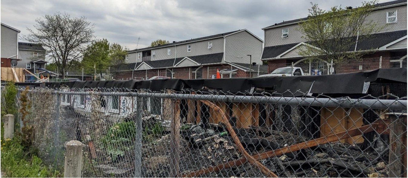
Figure 4: The demolished building of Block 3 in the foreground, with the subject site in the background
