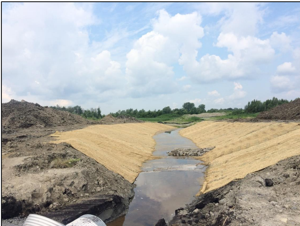
Photo 6: Water in drainage ditch at Cambrian Road crossing in July 2017.
