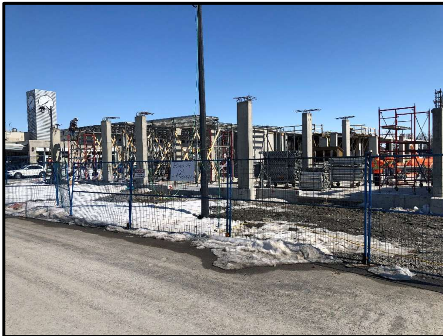
Photograph 2: View of the residential/commercial building under construction on the north portion of 2 Modugno Place, facing east.
