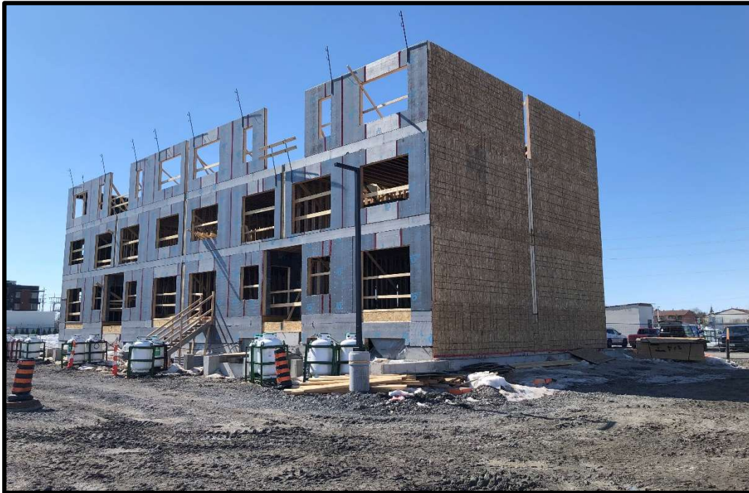
Photograph 1: View of the residential building under construction on the south portion of 2 Modugno Place, facing west.
