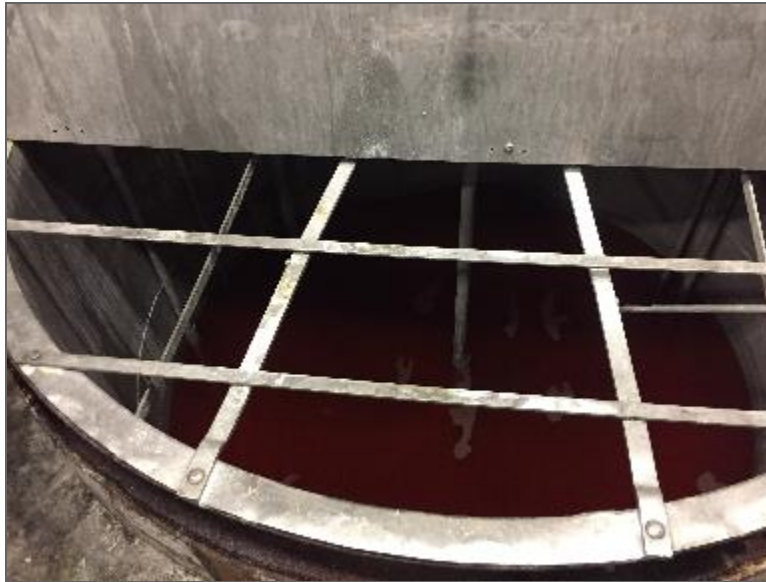
Photo 7 – Holding tank within Site Building B (collection of wastewater from trenches in the manufacturing area).
