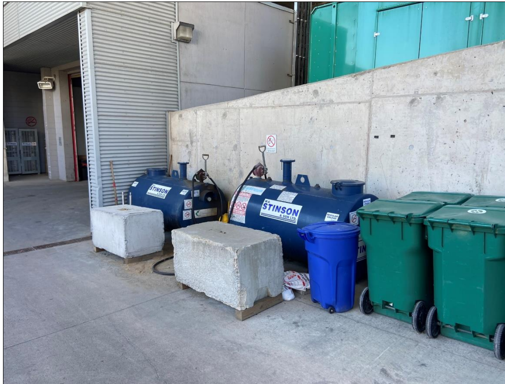
Photo 11: 500 L capacity coloured diesel and gasoline above ground storage tanks located on the ramp outside the loading dock area. Note: fuel spills would flow down the ramp to the grate floor drain.
