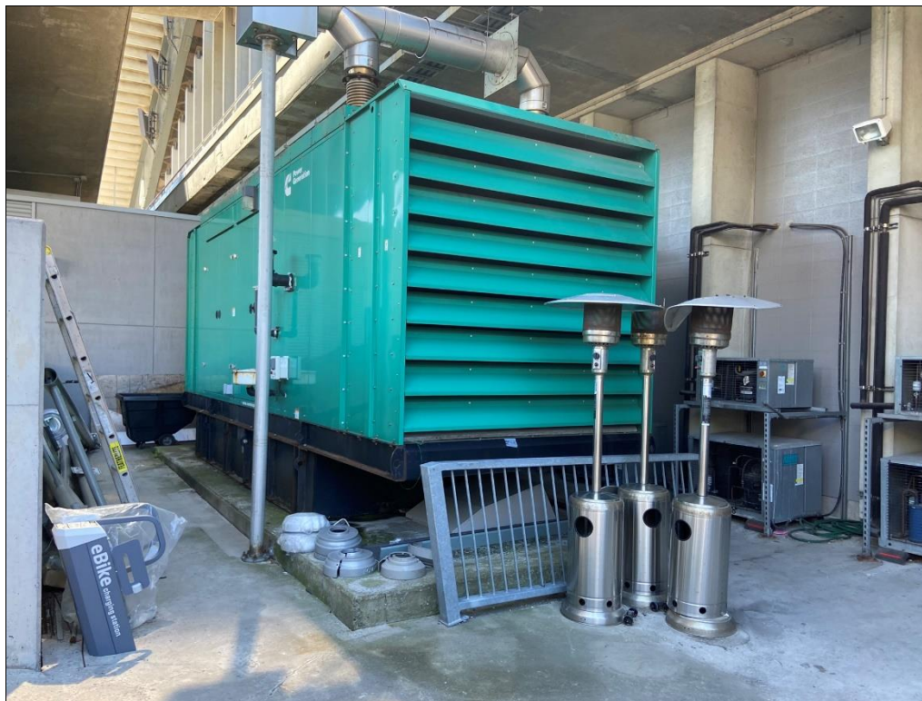
Photo 12: Back-up generator located outside the loading dock area on the east side of TD Place Stadium. Fitted with a 5,791 L capacity diesel storage tank.
