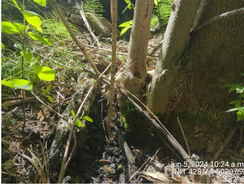
Photo 3: Tree in the channel resulting in steep of 22cm, downstream end of the culvert (June 5, 2024)
