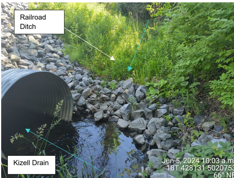
Photo 4: Rip rap at Kizell Drain creating a barrier at the downstream end of the ditch (June 5, 2024)
